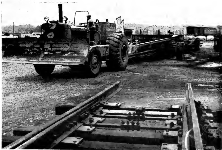
Giant carrier, drawn by tractor, is used to handle completed turnouts to storage and thence to site of installation.
